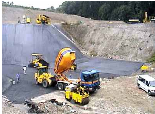
Fig. 6.3 Construction of the sanitary landfill Chrüzlen near Oetwil am See, ZH, in 1995 with a capacity of 600'000 t (Chrüzlen 2002).
