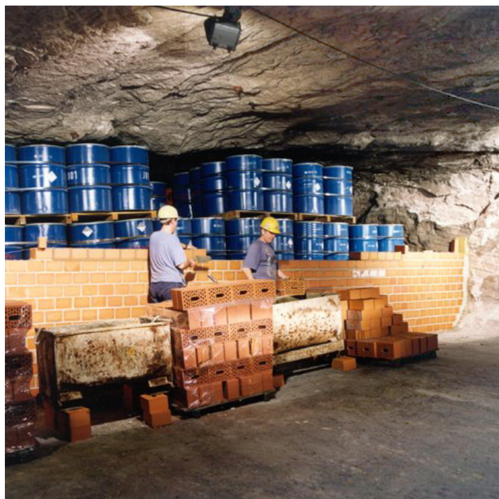
Fig. 5.5 Separation of one completed compartment by a brick wall in the underground deposit Herfa-Neurode. At the ceiling the rock salt vein is visible 11
