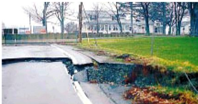
Fig. 10.2 Surface damages from the 1994 collapse of the Retsof salt mine, Genesee Valley, USA (Kappel et al. 1998)
